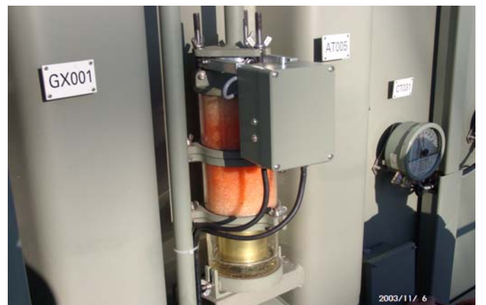
Fig. 3 Comparative measurements at a power transformer with a measuring flange for conventional dehydrating breathers (MESSKO, Oberusel)
